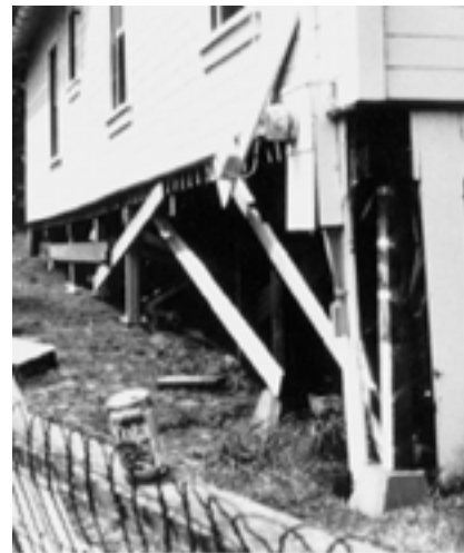
Figure 18 - The pier-and-post foundation under this home shifted during a recent earthquake.
